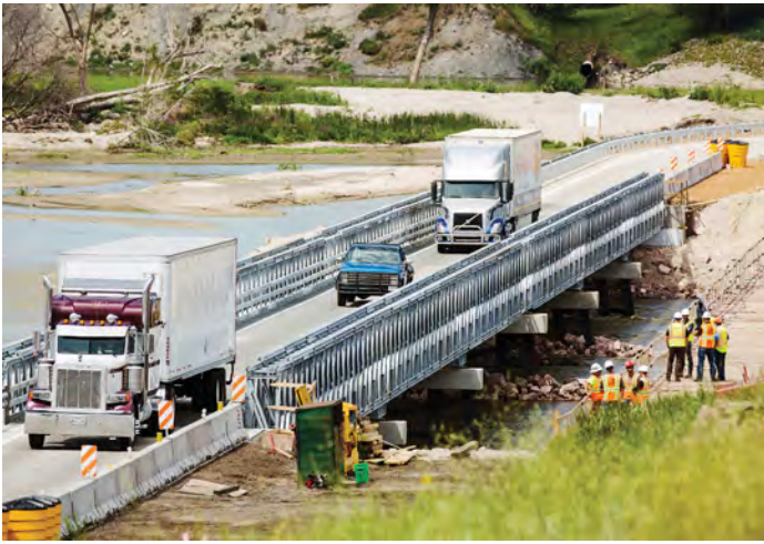
A temporary bridge structure was used on Highway 281 by Spencer, Neb. (Photo provided)
