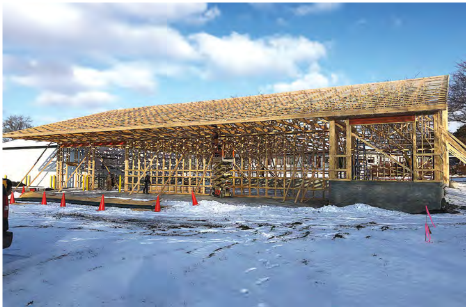
ABOVE: Construction is underway on a new 60-by-100-foot building. It marks the 13th building addition that Blackburn has undertaken. (Photo provided)
