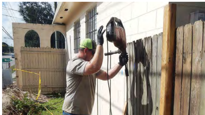
The affected resident's wooden fence was removed and stored for reinstallation after the project's completion. (Photo provided)
