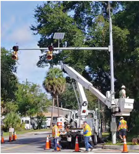
Gainesville, Fla.'s, Department of Mobility staff installs smart traffic devices at a local intersection. (Photo provided)
