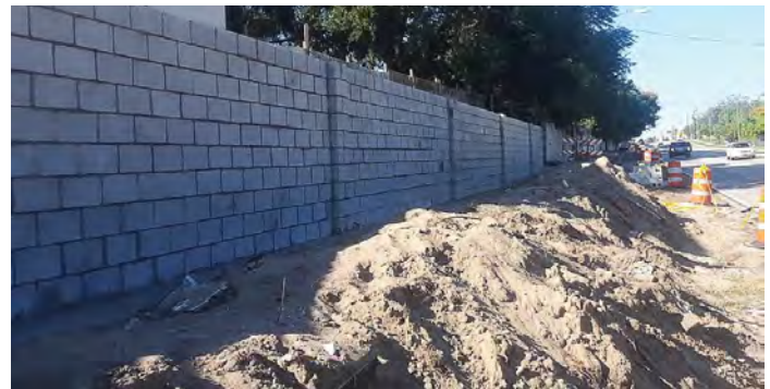
The existing wall/footer was demolished for an 8-inch-wide cantilever reinforced masonry wall. (Photo provided)
