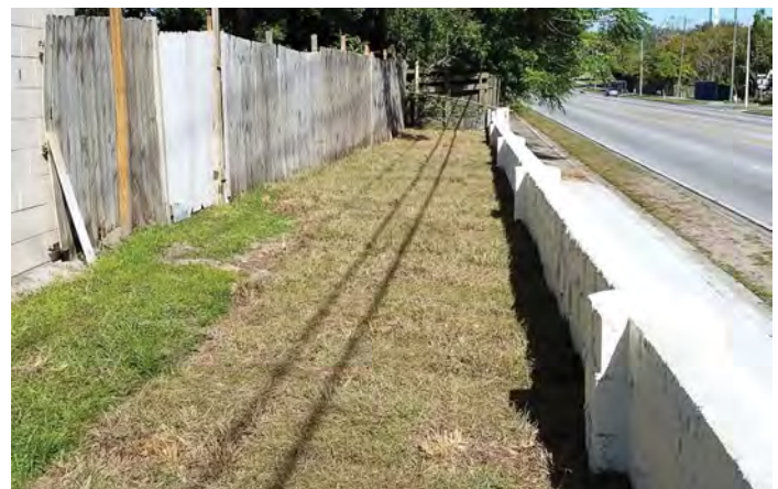
Following construction, the resident's yard was reinstated where it'd been disturbed. (Photo provided)
