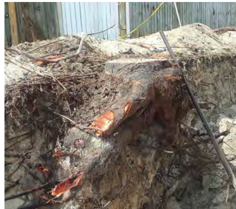
The project required the tree and its root system to be removed; the removal hole was then later backfilled. (Photo provided)
