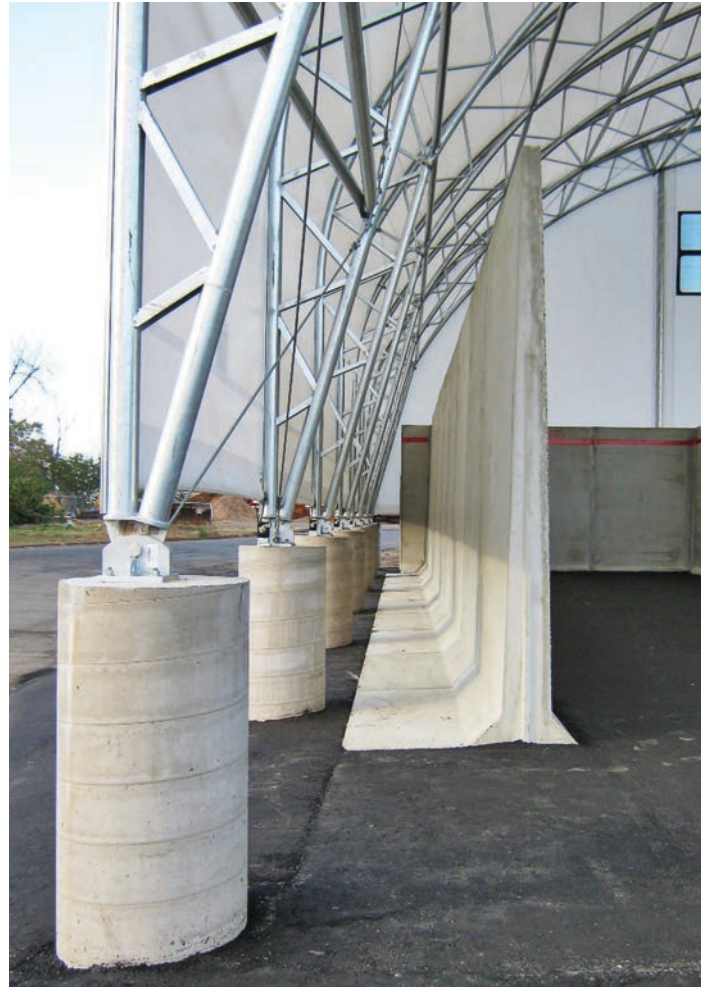
This is an example of Greystone’s design for independent building foundations and pre-cast walls. (Photo provided)
