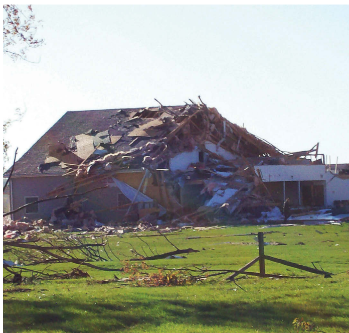
This is just one of the many homes damaged by the EF3 tornado that struck Nappanee after 10 p.m. on a Thursday night in October 2007. (Photo provided by Nappanee Fire Department)
