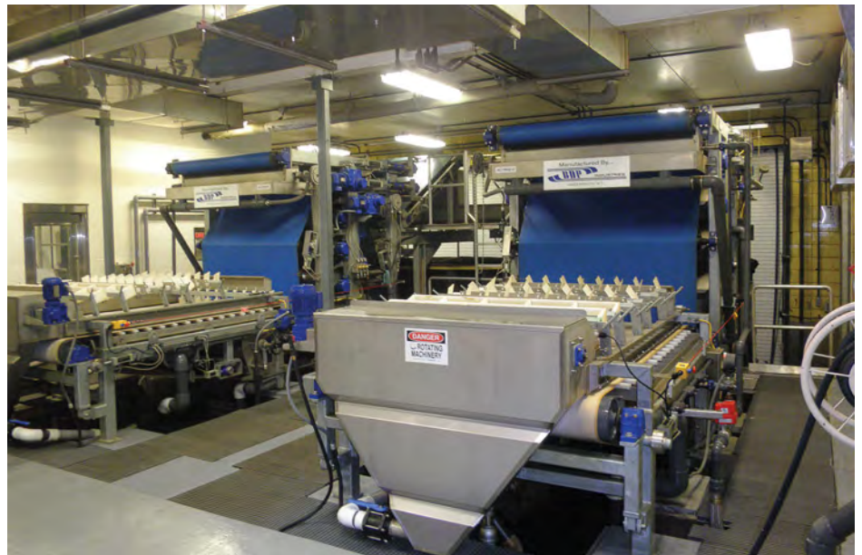
Community members are welcome to tour the Great Barrington Wastewater Treatment Plant, with Ely noting it'd be a great idea for environmental students who just might find an unexpected career path. (Photo provided)
