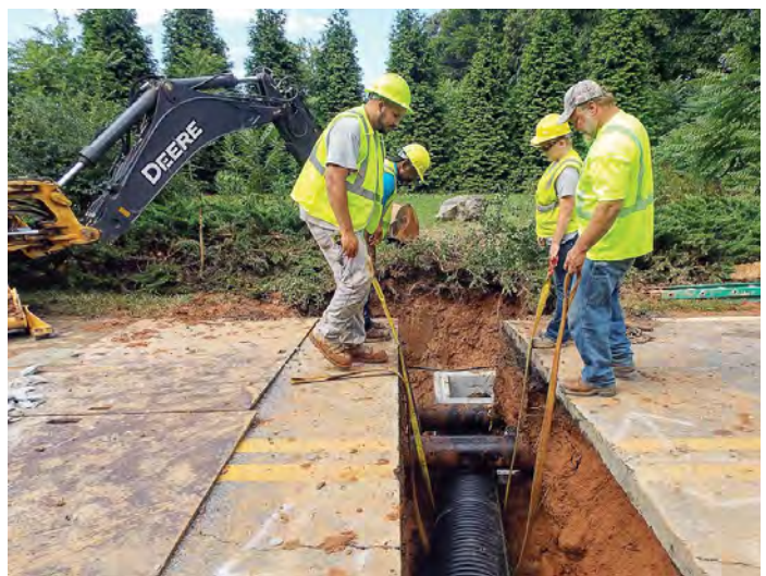
Asheville public works employees lower a pipe as part of a stormwater project. The department currently has a 9.5% vacancy rate. (Photo provided)
