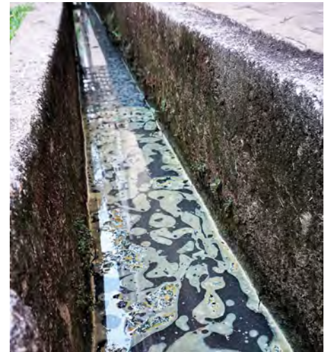
If food establishments and residents do not follow best practices or the F.O.G. ordinance, it can lead to disgusting or even hazardous consequences that affect the entire city. Oil and grease floating on top of the water in an open city drain is just one consequence of noncompliance. (Shutterstock.com)
