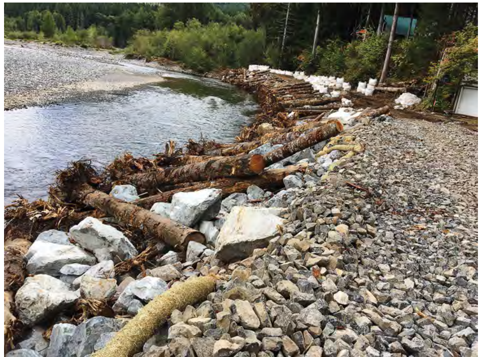
The award-winning Cowlitz River Erosion Project used stone and logs to protect the bank from erosion. The contractor used a local lumber source for the project, which saved the county money on transportation costs. (Photo provided)
