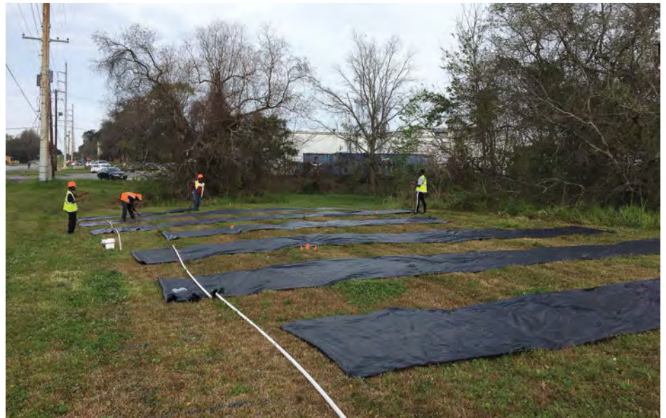
Skills imparted to interns include clearing land, identifying different tree species, installing drip irrigation systems and managing the trees as they grow. (Photo provided)
