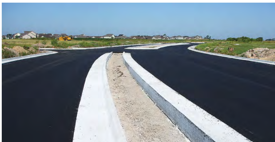
As research continues, there is hope of increasing the amount of recyclable materials used in roadways and bridges. Products that don’t require extensive durability, such as silt fences for runoff, could utilize a good amount of recycled material. (Photo provided)
