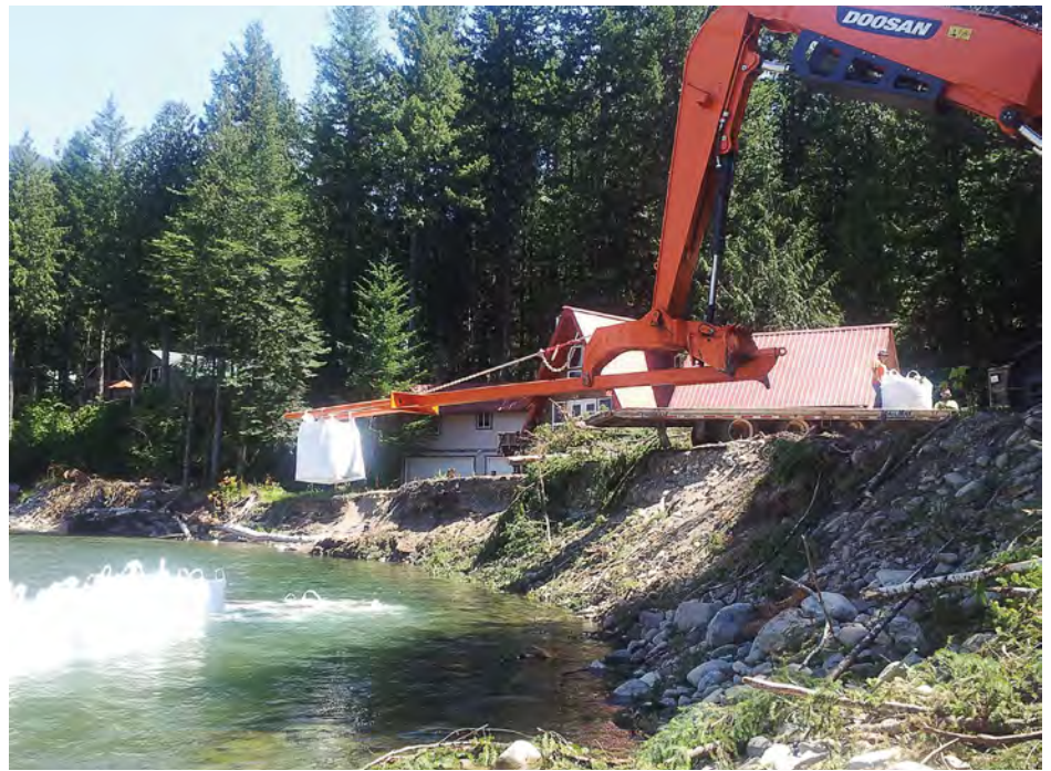
Work to combat erosion along the Cowlitz River started during the summer of 2018, first creating a barrier to the river’s current. (Photo provided)
