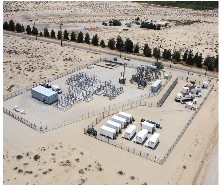
Resiliency is a major draw to microgrids. When the grid goes down, the microgrid disconnects from the main grid to supply backup power to one or more customers. Pictured is an aerial shot of the Borrego Springs microgrid. (Photo provided by SDG&E)
