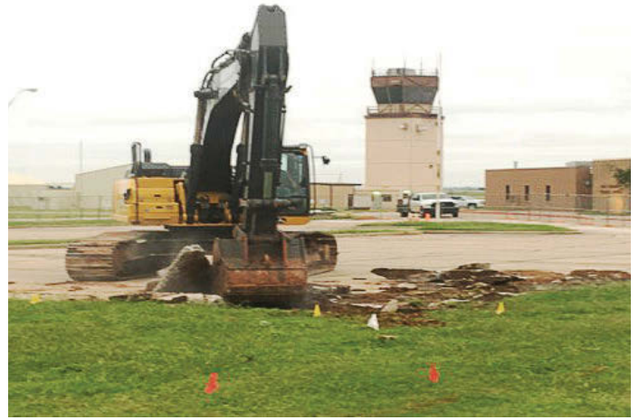
Ground was broken for the new terminal in September of last year, and work is expected to be concluded in mid-June. (Photo provided)
