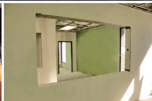
Public Defender's Office - used as drywall
