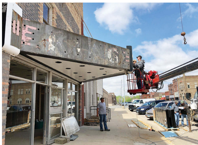
The old marquee is removed from Ida Grove, Iowa's, King Theatre. The city, seeing the value of a downtown movie theater, took over ownership of the King and has been renovating it. (Photo provided)
