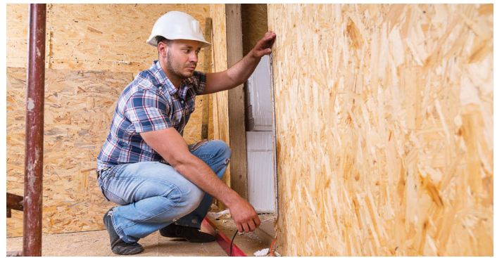
Contractors who partner with local unions participating in the S.T.E.P. not only get the benefit of local, qualified workers, but also have, at minimum, a portion of their Detroit Workforce Fund contribution waived. (Shutterstock.com)
