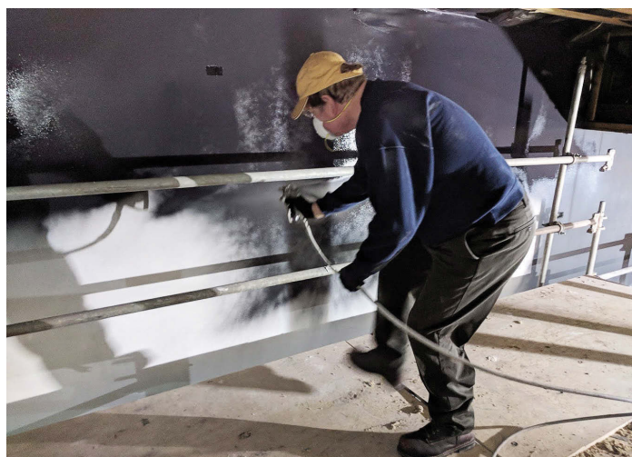
Black paint is applied to King Theatre's interior as part of the renovation process. (Photo provided)
