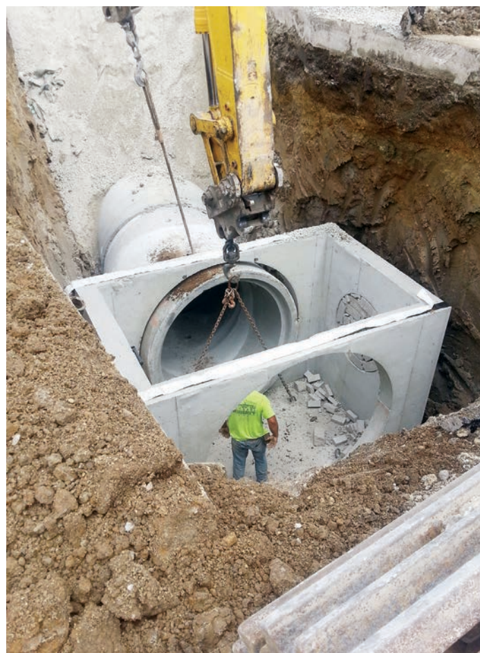
A worker oversees the placement of one component for Niles' updated Cleveland Street storm sewer system. (Photo provided)
