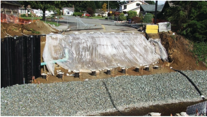
The natural material used in the bottoms of the updated culverts were all specified by the Washington State Department of Fish and Wildlife. (Photo provided)
