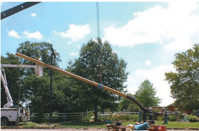
Workers from Bolin Enterprises are dwarfed by the 60-foot pitchfork as they install it on a farm property just outside of town. (Photo provided)
