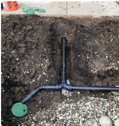
Pictured is a branched drain gray water system being installed in a yard in Davis, Calif. It will provide irrigation to the lawn. (Photo provided by EcoAssistant)
