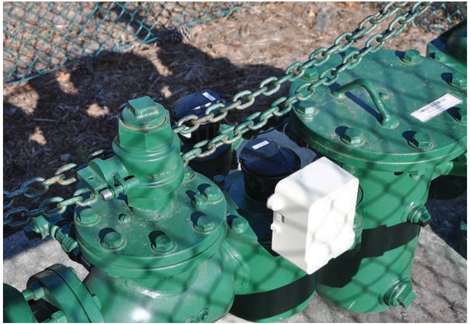
Pictured is a 4-inch Neptune FM meter, which is connected to a Sensus MXU. The Sensus MXU will retrieve the readings from the Neptune water meter and transmit them to a tower where the data will be passed to a database.” (Photo provided by Lakeland Water Utilities)
