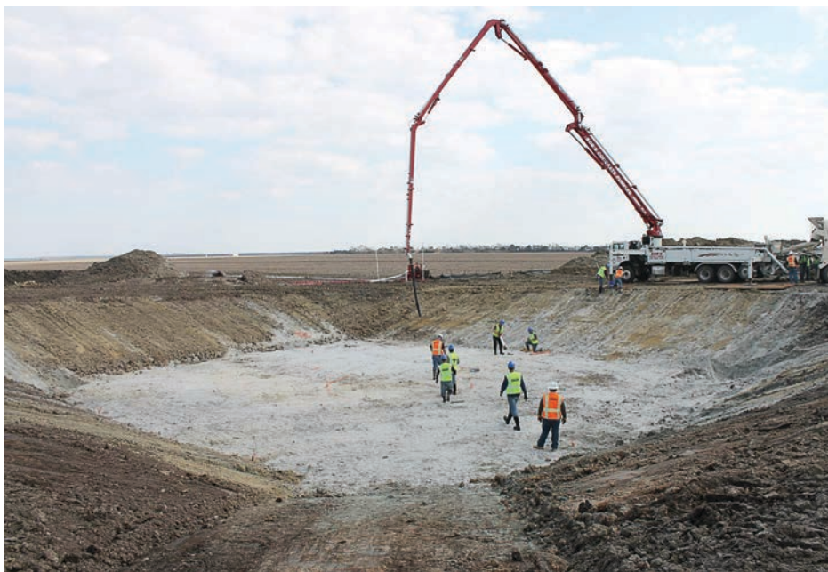
Construction of the Desert Wind Farm in Pasquotank County, N.C. While the turbines only take up a fraction of space on the land, much construction takes place. (Photo provided)
