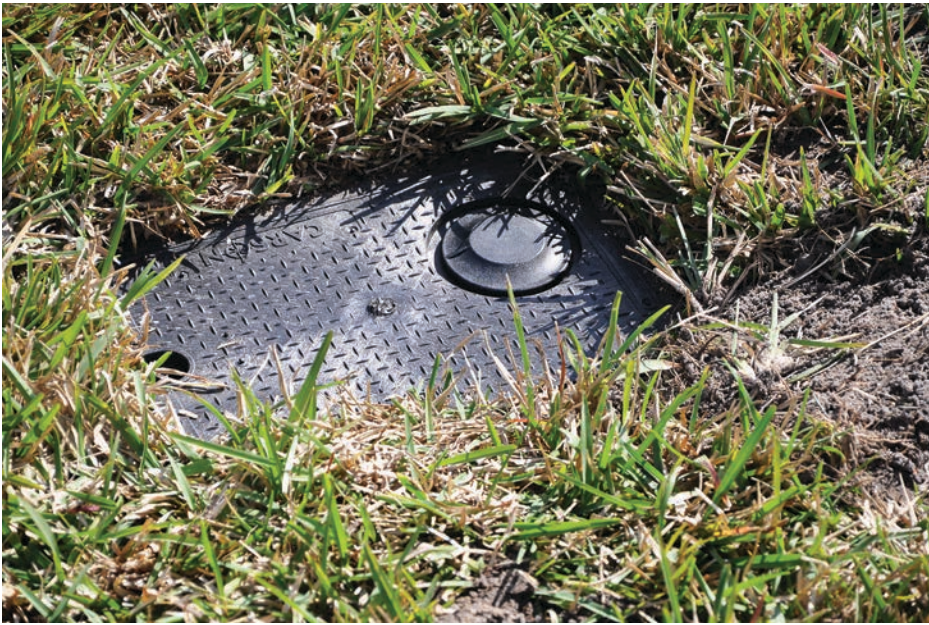
This photo shows the completed AMI installation, with only the MXU's transmitter being visible above the ground. (Photo provided by Lakeland Water Utilities)
