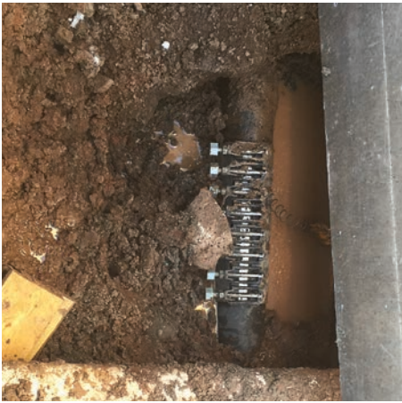
One of several repairs made by the city of Duluth. A wide array of technology is available today, giving cities the ability to specifically locate hairline fractures in pipes and listen for disturbances that would lead to a leak. (Photo provided)
