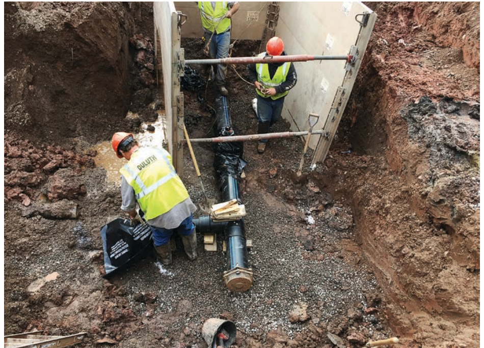
As stated by Chief of Utilities Eric Shaffer, 1 percent of piping should be replaced per year in Duluth, Minn. If not, then the city is falling behind. (Photo provided)
