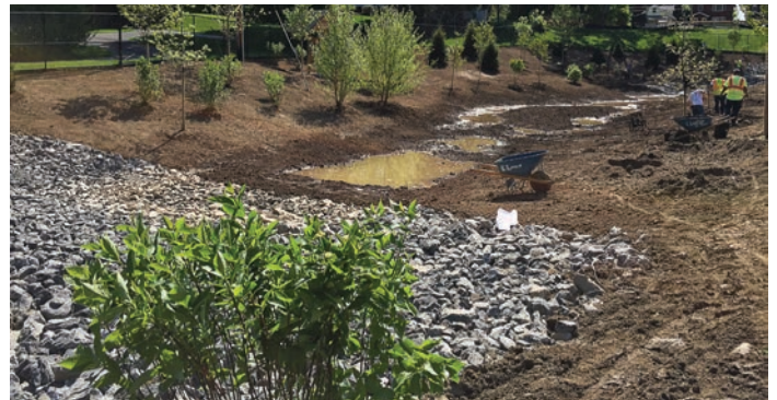
Construction of the created wetland in Albany was ongoing in this photo and water was already starting to collect. The wetland was part of a two-part solution to mitigate flooding in a neighborhood of the city that fell victim many times to “horrific flooding.” The city also installed an underground detention gallery under a baseball field in the neighborhood. (Photo provided)
