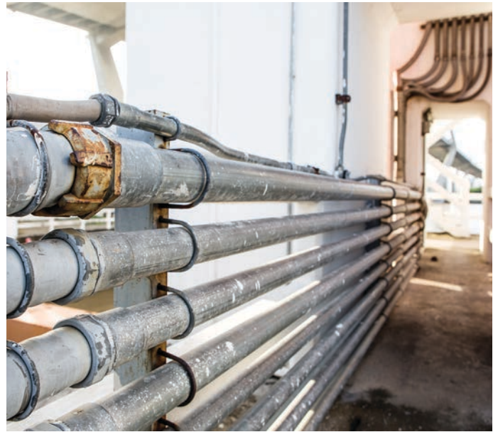
To avoid future issues with abandoned utilities, communicate to all parties and get in contact with the state's 811 organization to become better informed. (Shutterstock.com)
