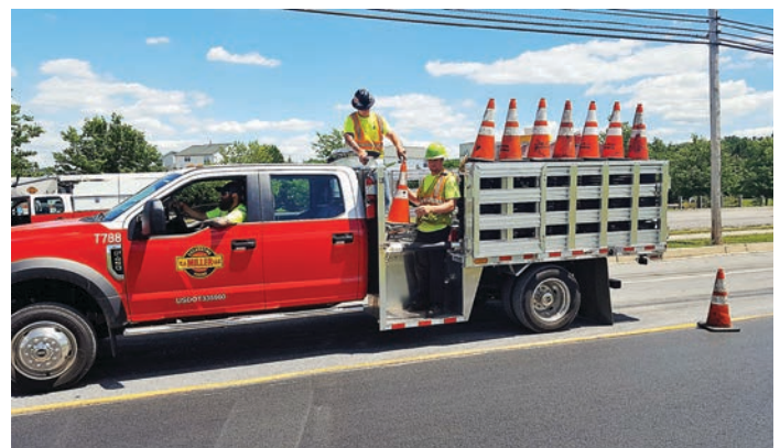
ABOVE: Workers place traffic cones from their stake body truck with a pulpit. EBY's investment in state-of-the-art technology allows it to customized available options to fit specific needs. (Photo provided)
