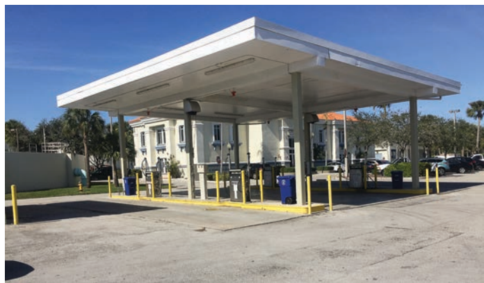
Miramar, Fla., has its own fuel depot that has 14 dispensers. Having the capacity to keep city vehicles running is critical during an emergency situation. (Photo provided)
