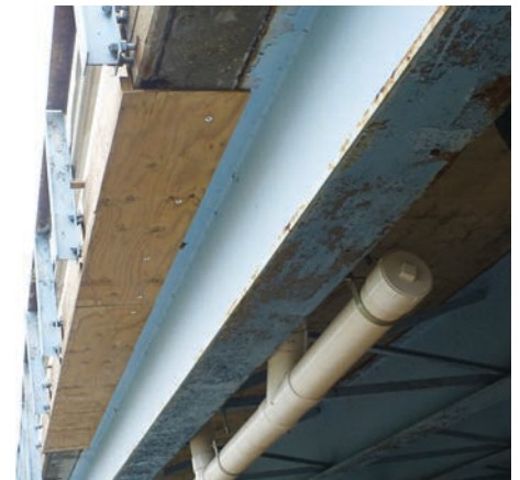
Plywood was used to prevent debris from falling on the bike path below prior to the construction of a new bridge. (Photo provided)
