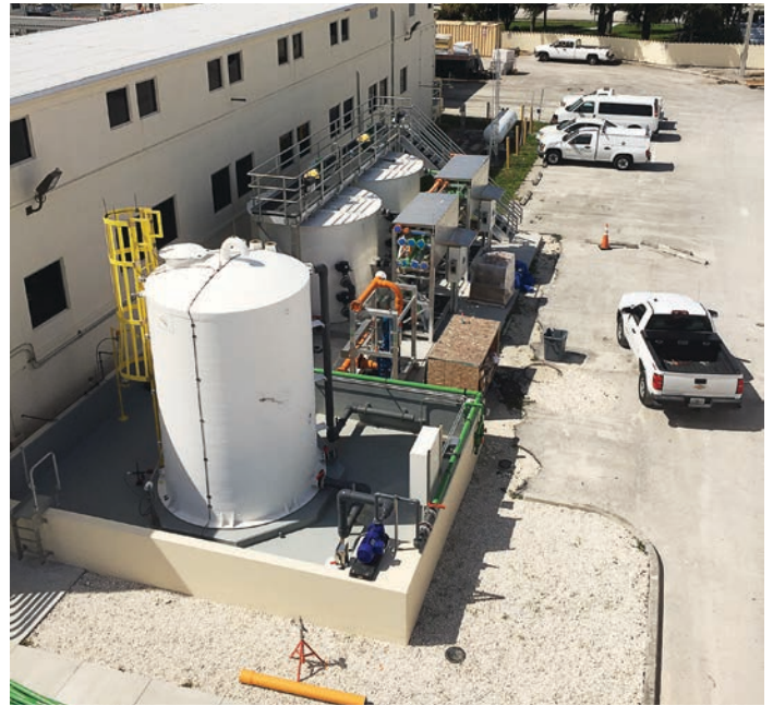
Basing the design off the nearby Palm Beach County Water Treatment Plant, Boynton Beach enhanced and optimized the contactor design. This resin regeneration area shows the recycled brine tank and resin regeneration skids. (Photo provided)
