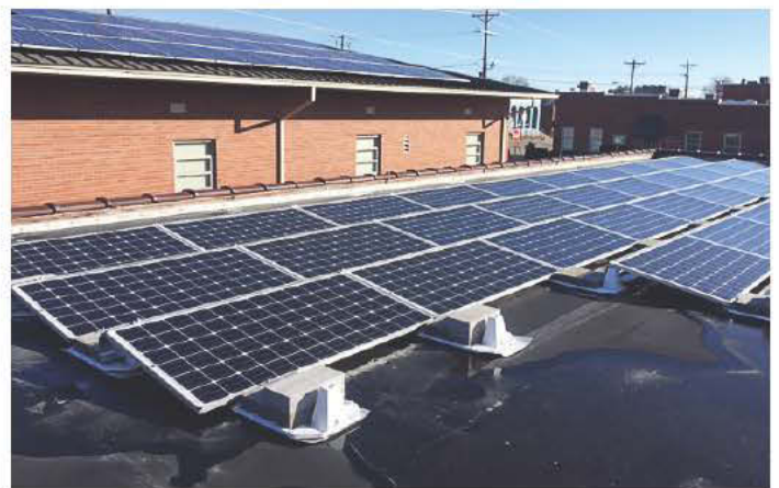
The town hall in Saluda, S.C., constantly sees citizens coming in and out, which brings more attention to the solar panels on top. (Photo provided)
