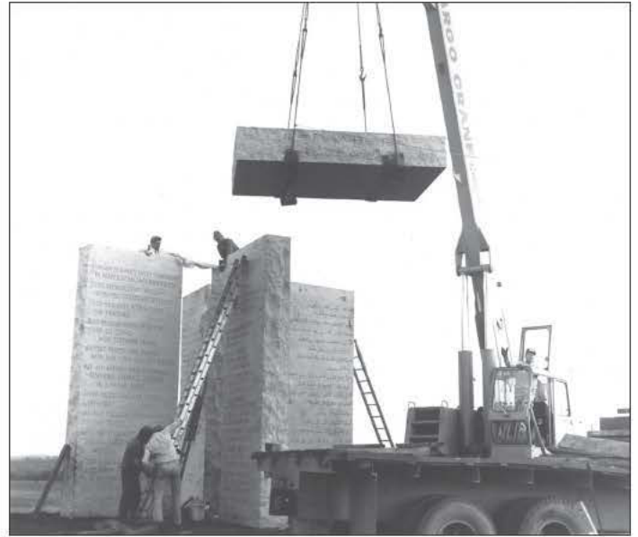
Workers carefully position the capstone onto the vertical pillars of the Georgia Guidestones. Drilled through the capstone is a slot enabling the daily noontime sun to illuminate the day of the year etched into one of the pillars. (Photo provided)
