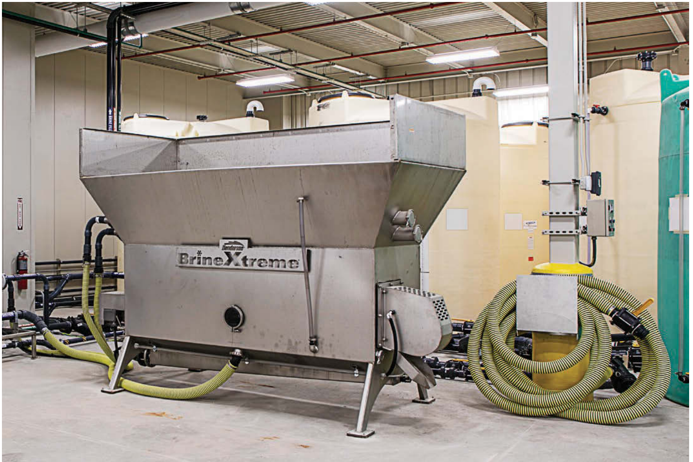
Farmington Hills's new automated brine manufacturing system has saved the city money on salt purchasing. The yellow hoses to the right are the fill stations. (Photo provided)
