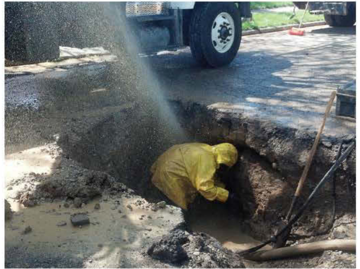
Middletown, Ohio, utility workers deal with a broken water main. A situation such as this could cause a worker to be overcome by the water and result in an accidental drowning. Middletown utility workers have increased training in all area of confined space safety after losing a co-worker in a 2010 atmospheric hazard. (Photo provided)
