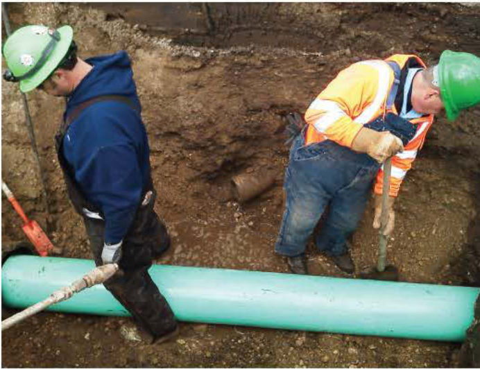
City of Middletown, Ohio, utility workers work on a sewer line repair in their city. The department lost one of its own in 2010 when Jabin Lakes was overcome by a gust of oxygen-depleted air after opening a manhole cover. (Photo provided)
