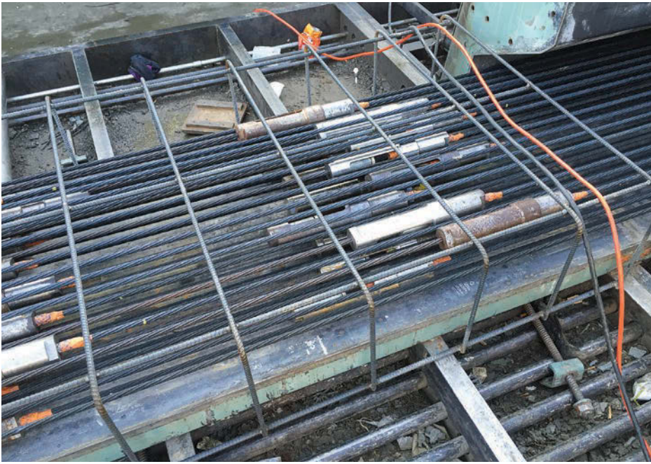
Carbon fiber strands provide many benefits to bridges as they are lightweight, non-corrosive and offer high tensile strength, which should extend the life of the bridge by 25 years or more. (Photo provided)
