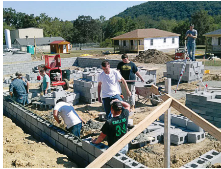
Students from Tazewell High School in Virginia work on a foundation. (Photo provided)
