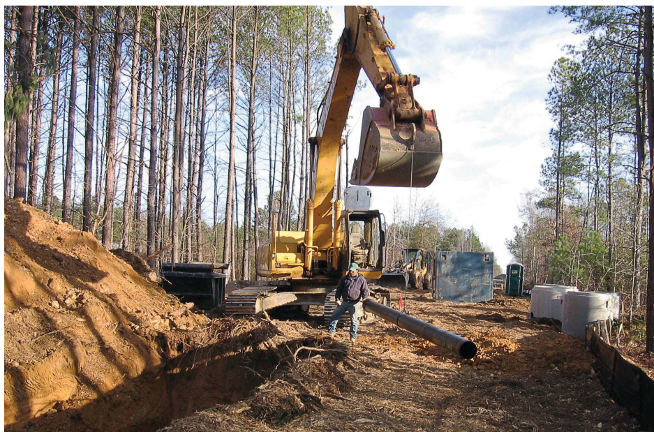
A public/public partnership with the city of Gainesville, city of Flowery Branch and the town of Braselton in regards to sewer service has been particularly beneficial for Oakwood, Ga. (Photo provided by city of Oakwood, Ga.)
