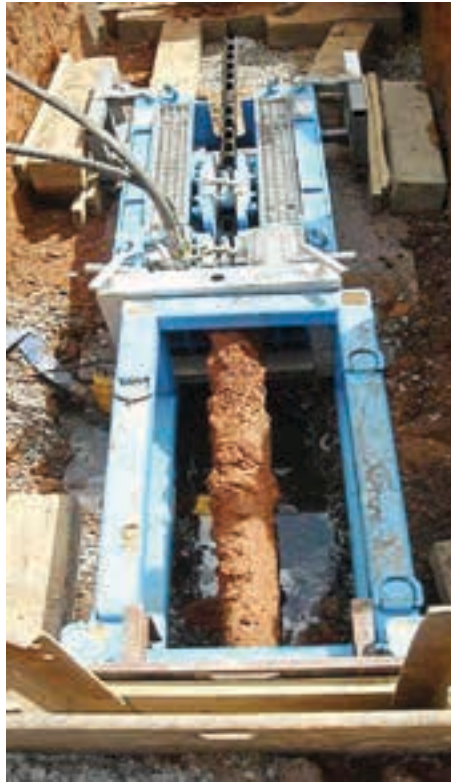
LEFT: A piece of the old cured-in-place pipe is pulled back into the pit on the pulling side of the process. There is a steel plate that breaks the CIP as it gets to the machine. (Photo provided)
