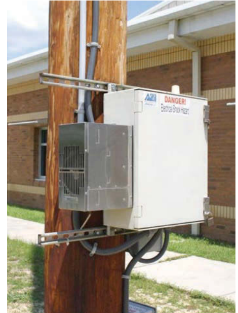
Multiple Jerome 651 units can be linked to form a perimeter monitoring system that continuously monitors H 2 S levels. (Photo provided)
