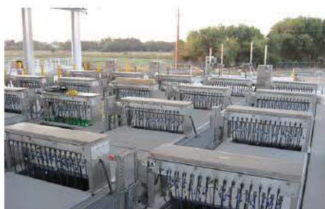
In California, the city of Roseville's Dry Creek Wastewater Treatment Plant has one of the largest LPHO systems ever designed to produce recycled water. (Photo provided)
