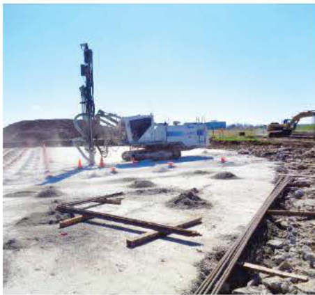
Tank construction to date includes the engineered fill on which the tank foundation will sit. (Photo provided)
