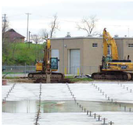
Vernon Azevedo, P.E., Remedial Measures Program manager in Lexington, said the rods sticking up through the engineered fill are rock anchors that are embedded into bedrock 22–25 feet deep. They will extend into the tank foundation to protect it from hydrostatic forces that could damage it. (Photo provided)
