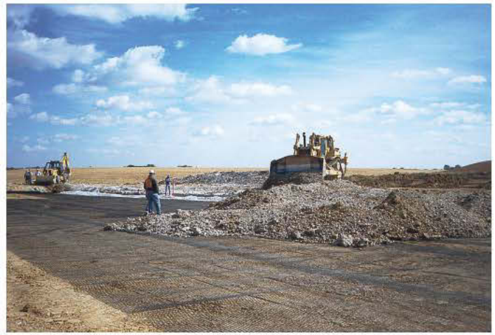
Hard-packed clay was excavated to construct the permanent disposal facility for the Weldon Spring chemical works site. The clay provided the foundation and cover for the 1.48 million cubic yards of radioactive waste buried in the cell, which is designed to keep the material entombed without leakage for 1,000 years. (Public Domain via Wikimedia Commons)
