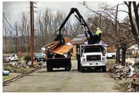
Another operator helps clean up post-tornado. (Photo provided by Mark Doerfler)
