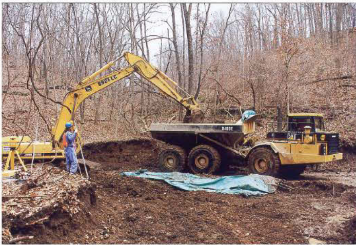
Workers remove soil from one of the drainage areas near the Weldon Spring site as part of the government's decontamination project. The decision was made to bury the contaminated remains of a uranium processing plant onsite rather than risk shipping the material to Utah or Washington state. (Public Domain via Wikimedia Commons)
